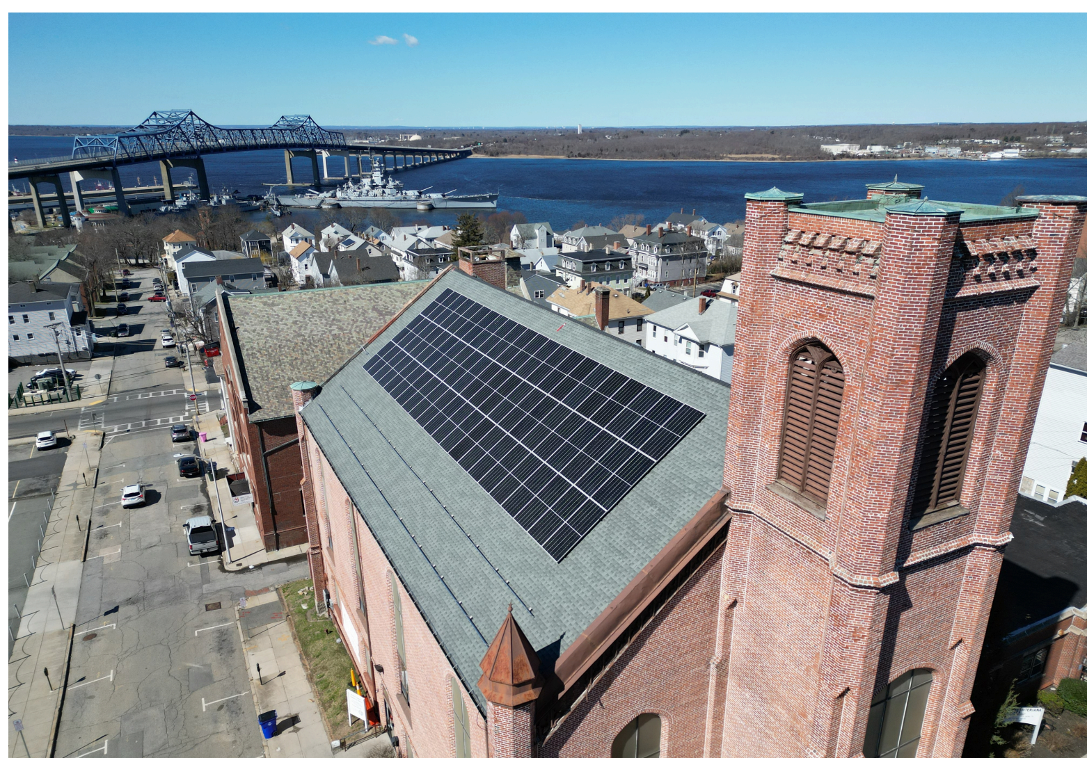
Image Credit: Sunwealth Power Inc.
